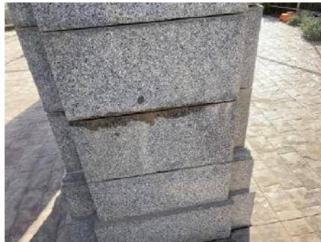
When joints were cleaned, trapped water drained out from within the the column
