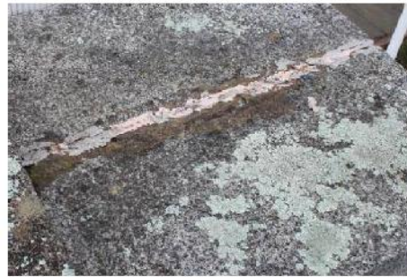
Poor quality mastic in joint allows water to enter the top of the memorial.
