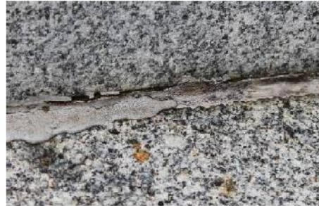
A combination of mastics has been used over time to try and seal the structure.
