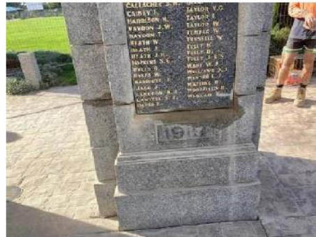
Trapped water draining from column on south side
