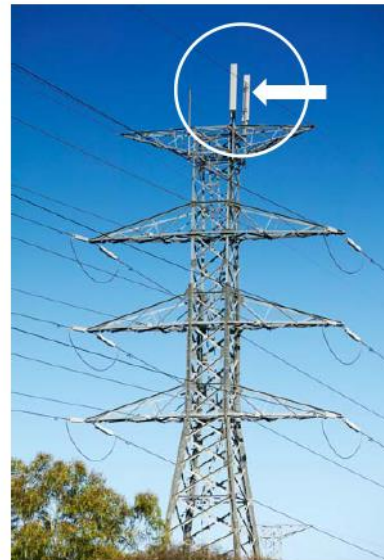
Macrocell base station antennas co-located on an existing high voltage tower.
