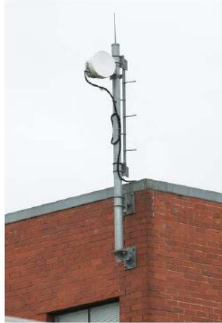
A radiocommunication dish used to send a radiofrequency signal from a macrocell base station to another base station (line-of-sight).
