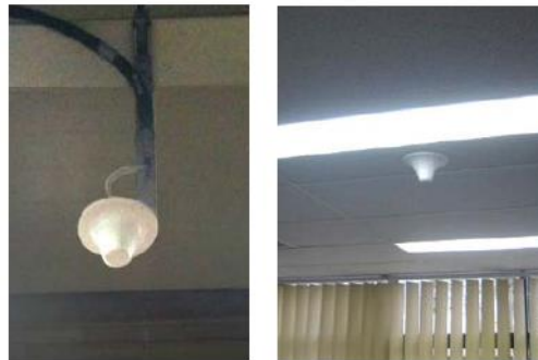
Left-right: Picocell antenna suspended from a ceiling; A cone shaped picocell on a ceiling.
