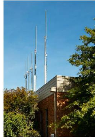
An array of omnidirectional antennas.
