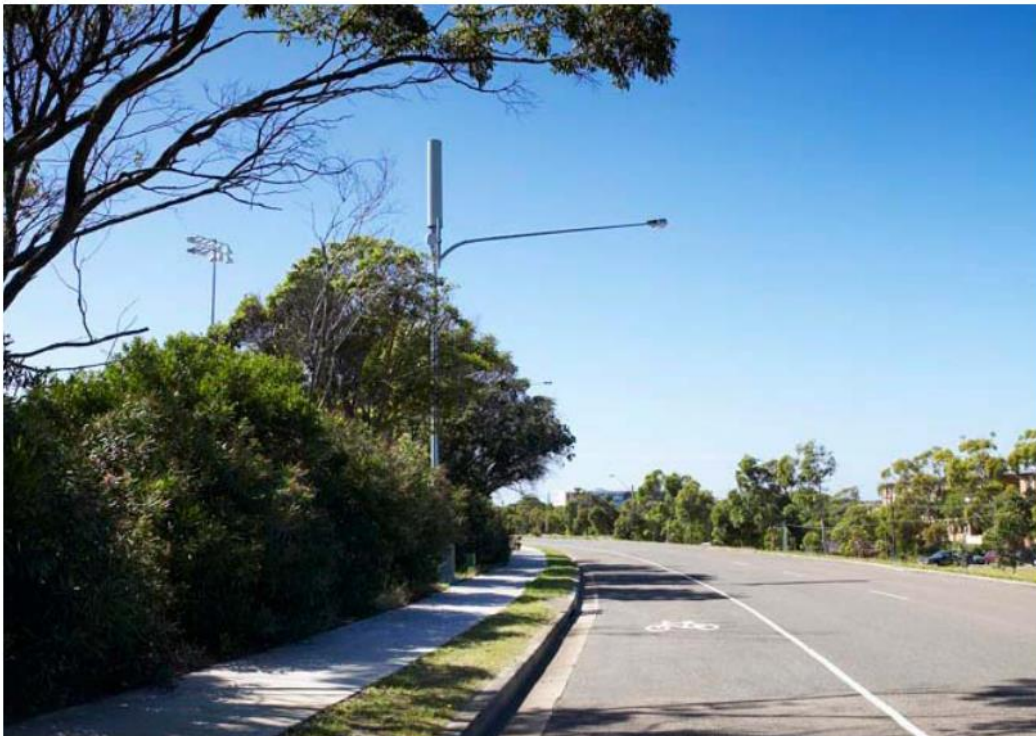
Panel antenna on street light pole
