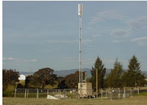
Temporary macrocell base station (consisting of two panel antennas) on lattice support mount deployed at a sporting event.
