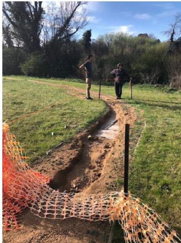
Photo 1. Damage to the pedestrian path along Bombay Road caused by heavy rain and wash. Note also the grass encroachment onto the path which is beyond the community volunteers to manage. A more water and weed resistant path surface would be ideal in this location but costs were beyond the grant resources that BULG was able to acquire.
