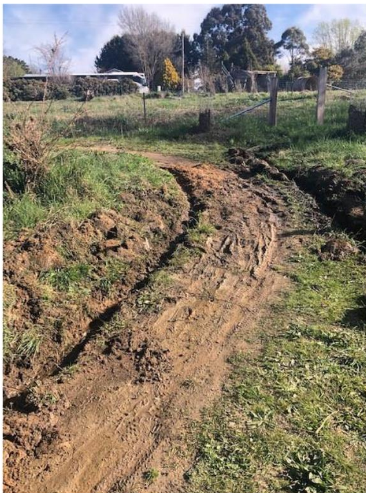
Photo 2. Section of the pedestrian path along Bombay Road (adjacent to the Community Gardens) that has been affected in recent years by continuous groundwater seepage. This has been a major impediment to all users with at least one person in a mobility scooter getting bogged in September 2020. While volunteers have trenched drains alongside the path this has had little impact. Resolution of this drainage issue is beyond the resources of the community group.
