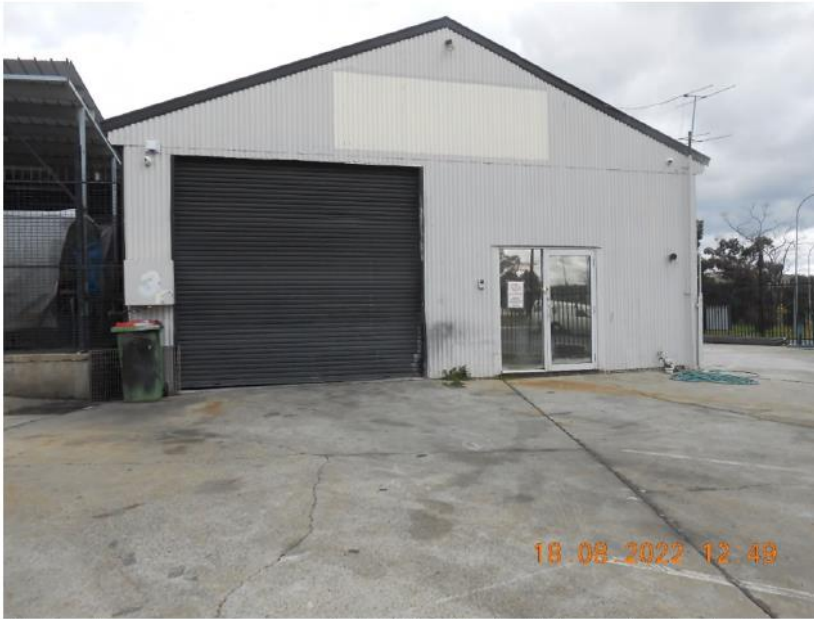
Photo shows access doors to building that will be restricted by the construction of the pole sign.
