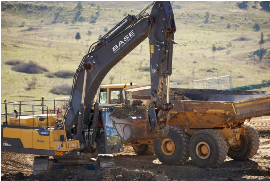
Figure 2 – From CJD Equipment’s testimonial showing BASE Construction branding on specific equipment sighted in Wickerslack Lane
