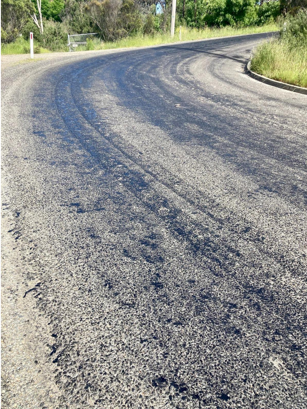
Figure 5 – Damage to Wickerslack Lane road surface, birth of the new La Brea Tar Pits. In the center of the photo is the entrance to my property at 133 Wickerslack.
