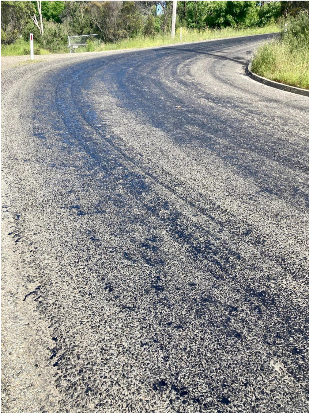
Figure 5 – Damage to Wickerslack Lane road surface
