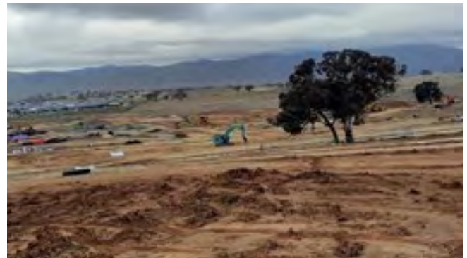
Poor erosion/sediment controls on subdivision site.
