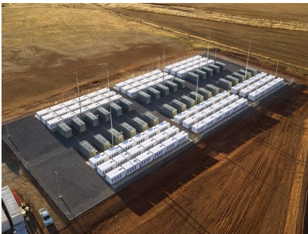
Figure 1 - Example of what a battery facility looks like
