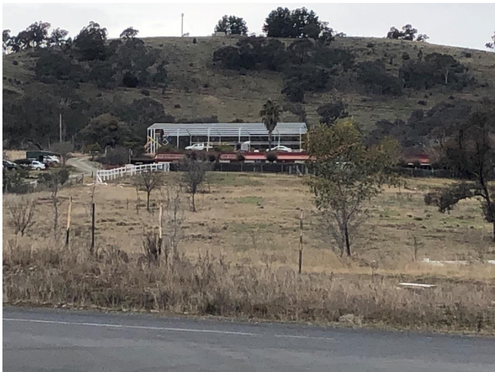
Figure 7: The Shed as Viewed from Fernleigh Drive, Having Begun Construction Without Approval.
