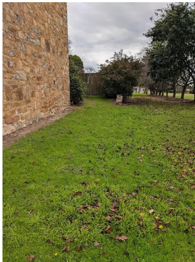
Figure 8 - Side of Museum showing constrained existing access to rear of the site
