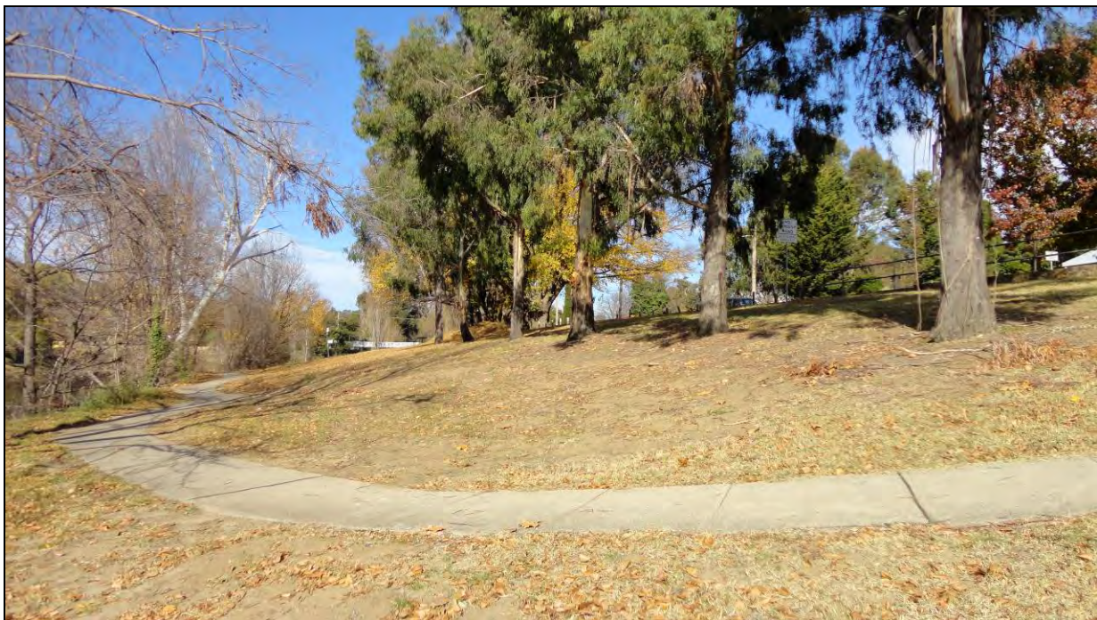
Photo: Minor soil erosion on slope between the river and southern end of Collett Street
