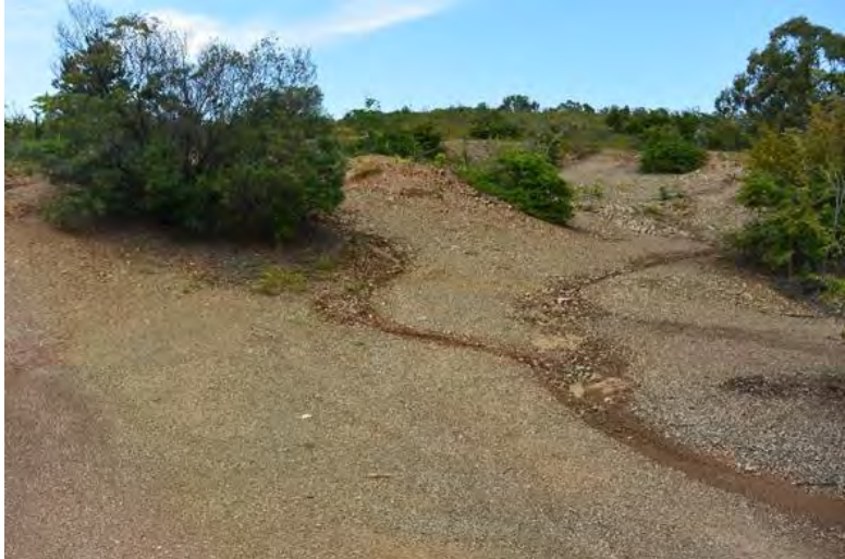
DSC 3790: Sheet and rill erosion across the quarry site
