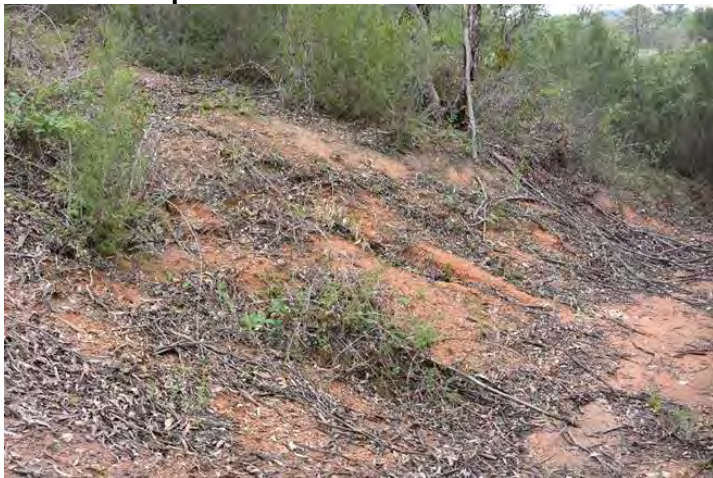
DSC 3777: Minor erosion on back batter of erosion control bank
