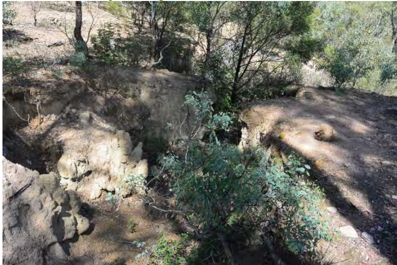
DSC 3810: Areas of eroding bank collapsing into creek bed
