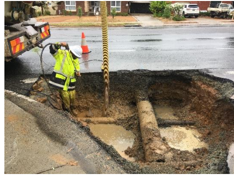
Photo 22: Cooma Street water main
