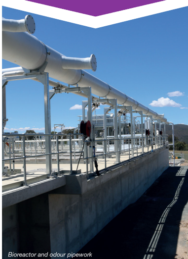
Bioreactor and odour pipework
