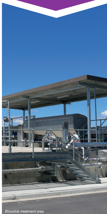
Biosolids treatment area
