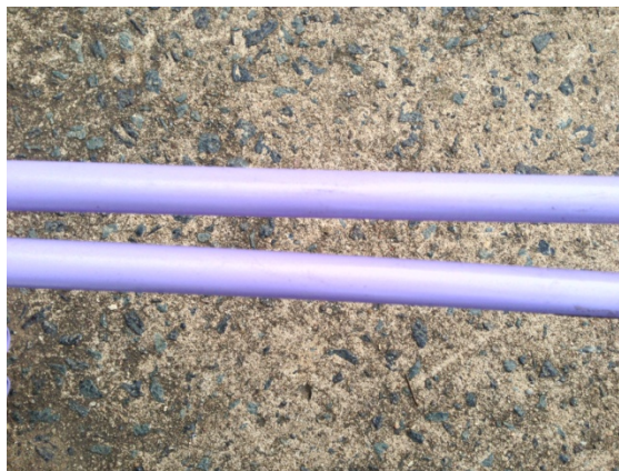
Figure 3: Non-drinking water pipe examples
